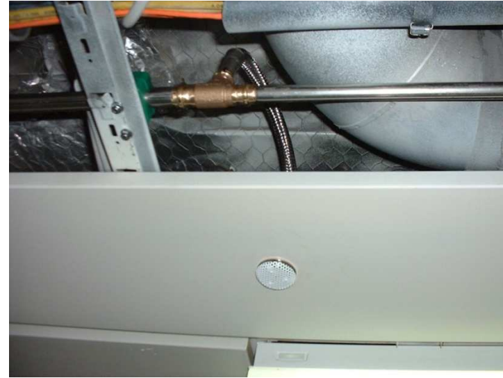
■ Concealed sprinkler with flex pipe
