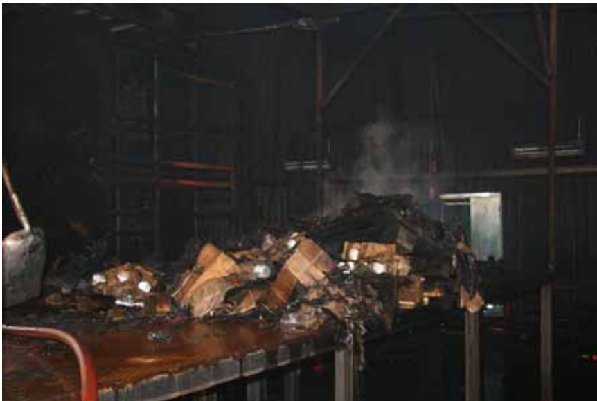
Figure A-159 Test 6S(HP-5.8): Fire damages as seen from the left hand side.
