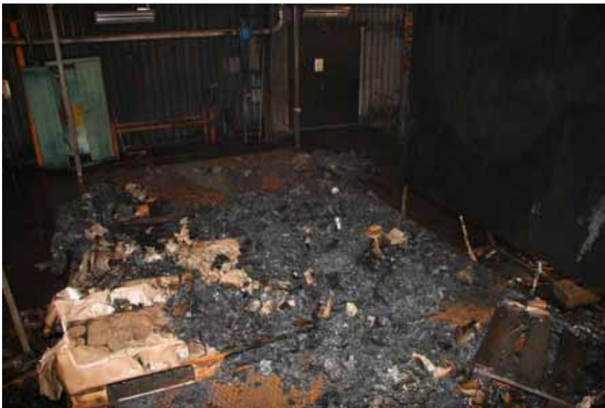
Figure A-140 Test 4S(5): The fire damages after the test. Almost all combustible material is consumed.
