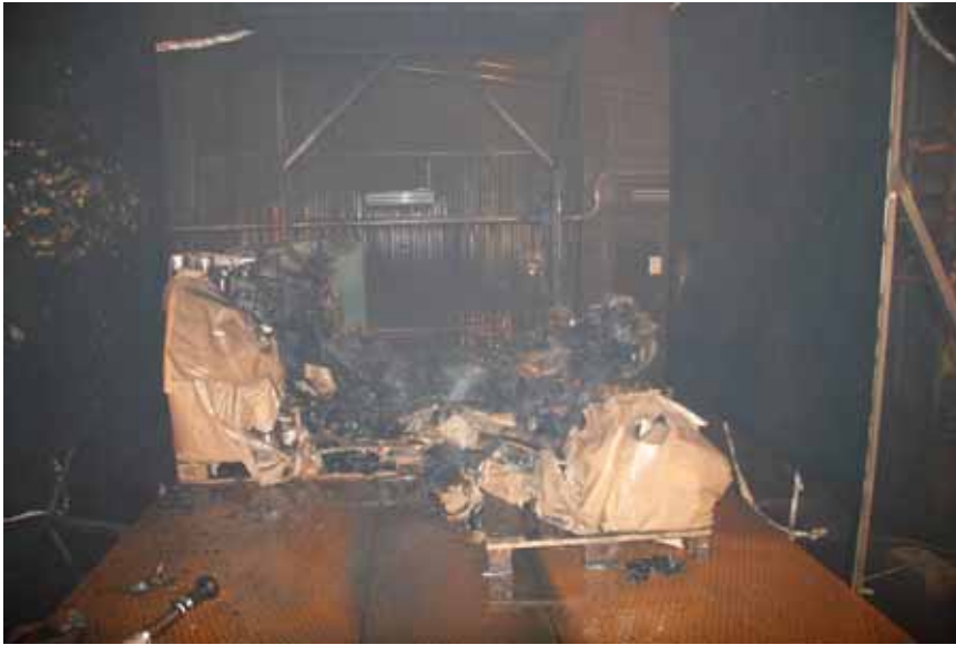
Figure A-151 Test 5S(15): The fire damages, as seen from back.
