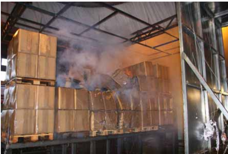
Figure A-32 Test 3E(10): Fire damages as seen from the right hand side.
