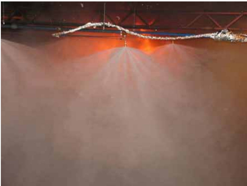
Figure A-66 Test 6E(HP-4.6): Photo at 01:50 [min:sec] after fire ignition, at full system operating pressure of the high-pressure water mist system.
