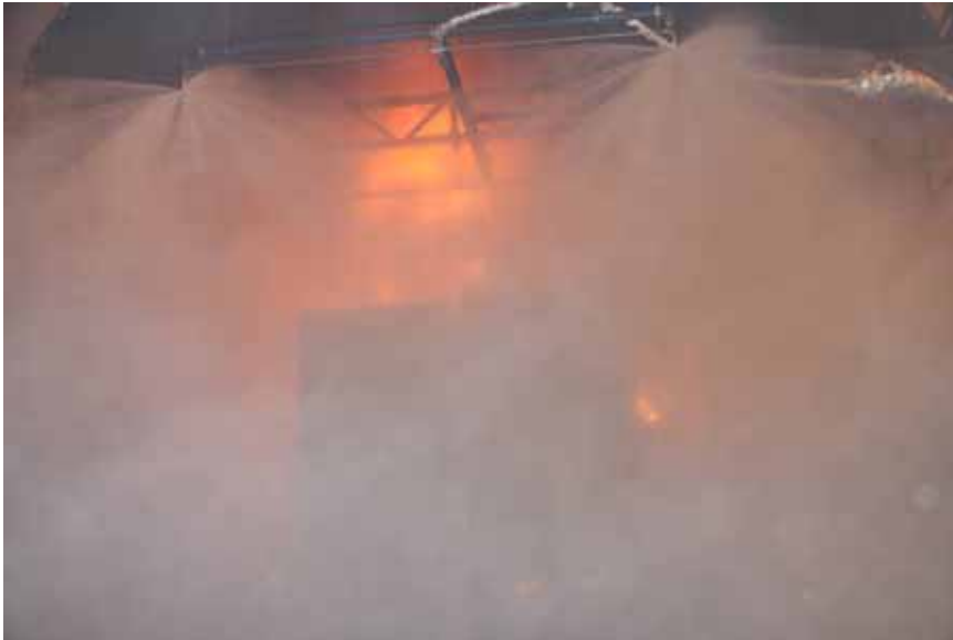
Figure A-67 Test 6E(HP-4.6): Photo at 04:50 [min:sec] after fire ignition, the fire increases in size. The fire is not controlled by the system and the test is terminated.
