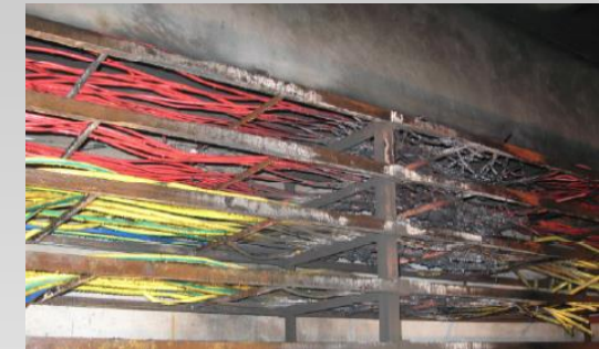
Fire damage after test
