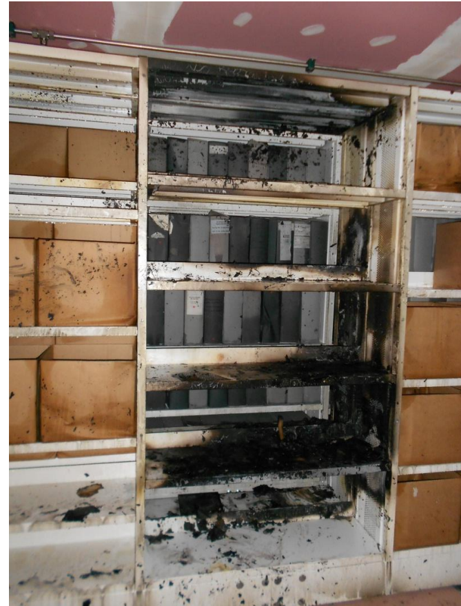
As cleared showing damage to only one section
