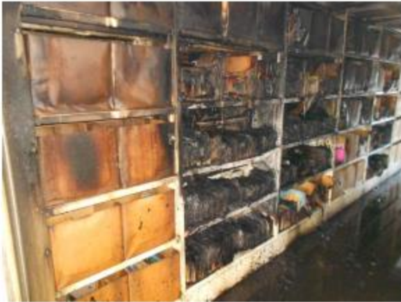
Test 2 - Row G Fire Damage
