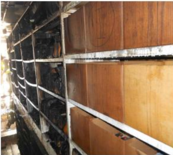
Test 2 - Row I Fire Damage
