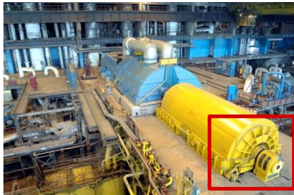
Turbine bearing including pressurized lubrication oil
