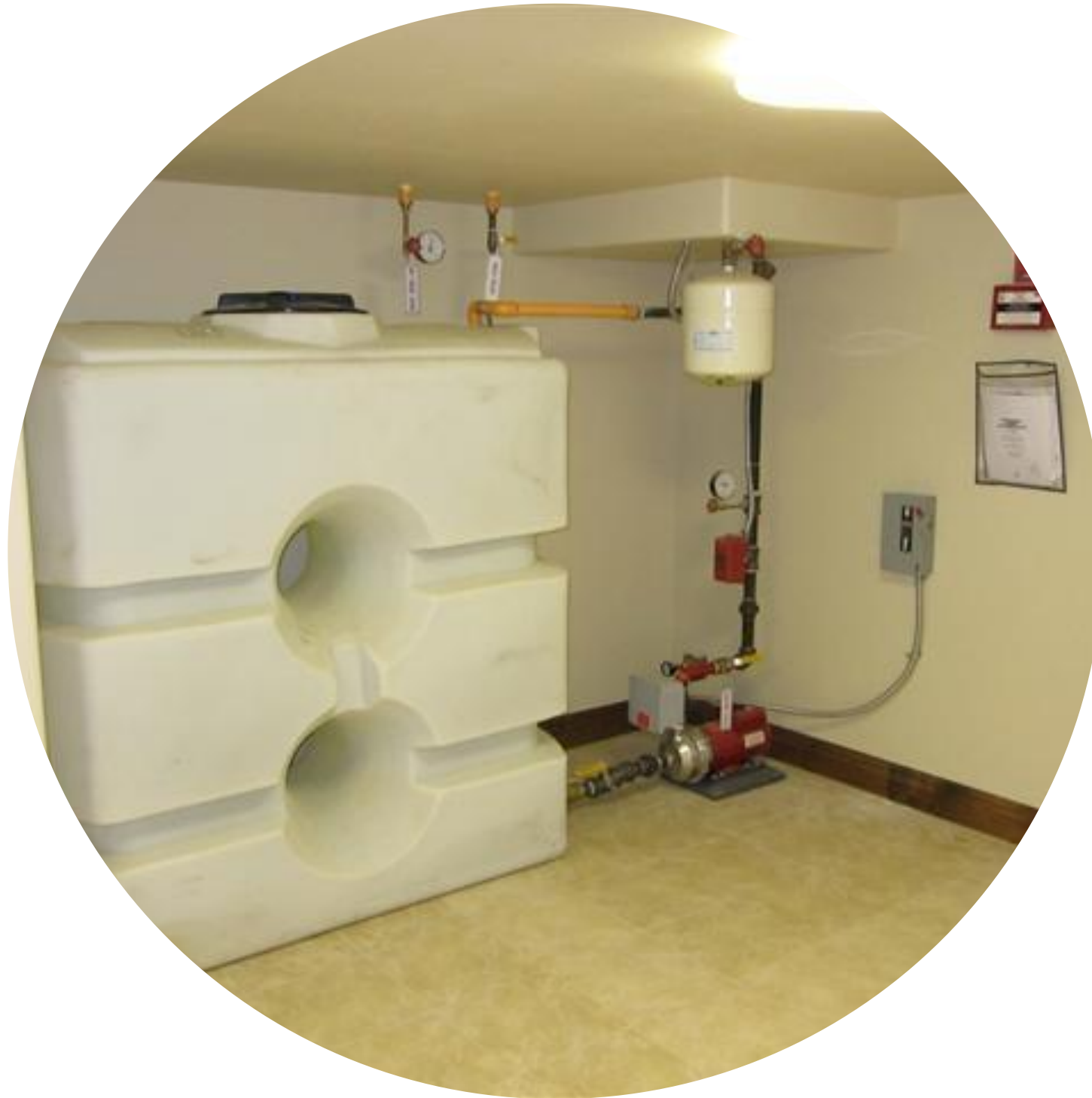
DIFFICULT TO RETROFIT
