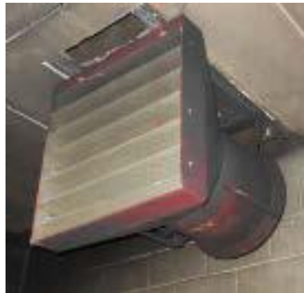
Fire protection devices
