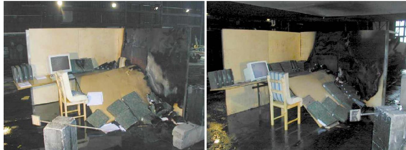
Fire damages after the worst test for both systems (left sprinkler system and right water mist HI-FOG)
