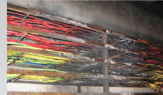
Fire damage after test
