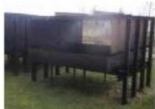
Fixed fire protection 37 Gary Howe reports on fire suppression for industrial oil cookers
