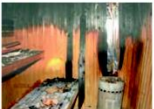
Sauna fires 15 Gary Howe and Stuart Lloyd investigate the use of water mist
