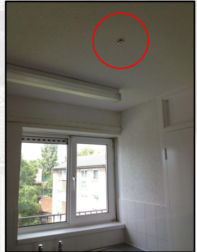
The Single Nozzle that activated is pictured above.
