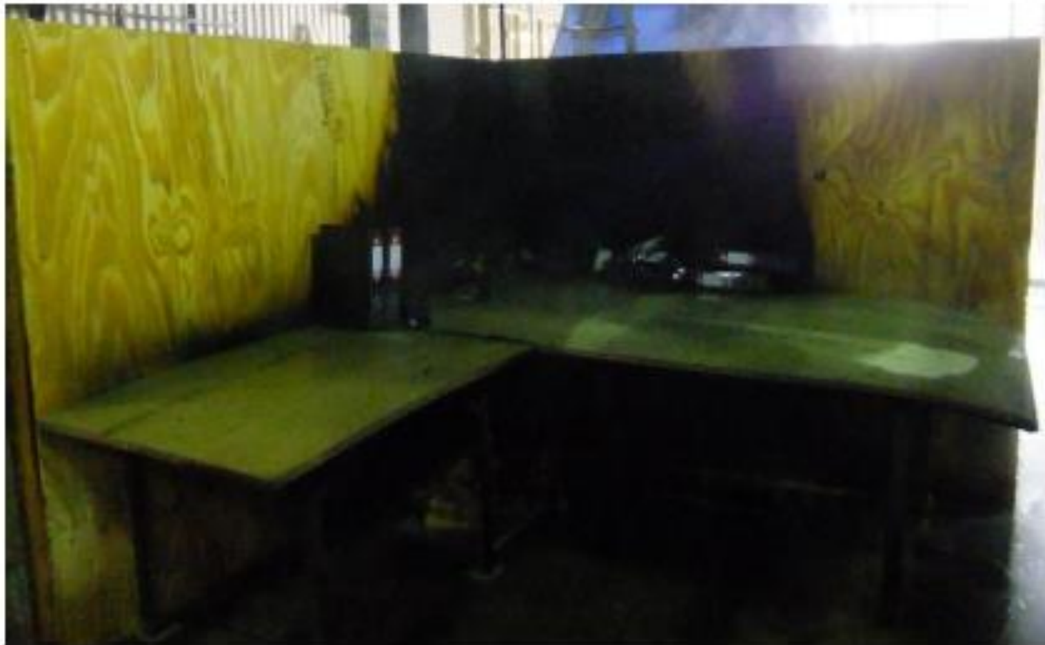
Figure 19 – Fire damage to the plywood walls, foam sheets and box files
