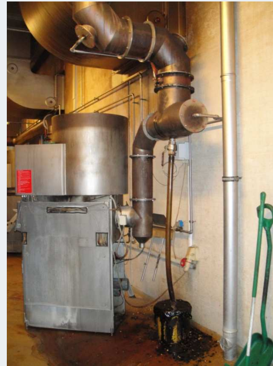
Tar dripping from the exhaust channel.
