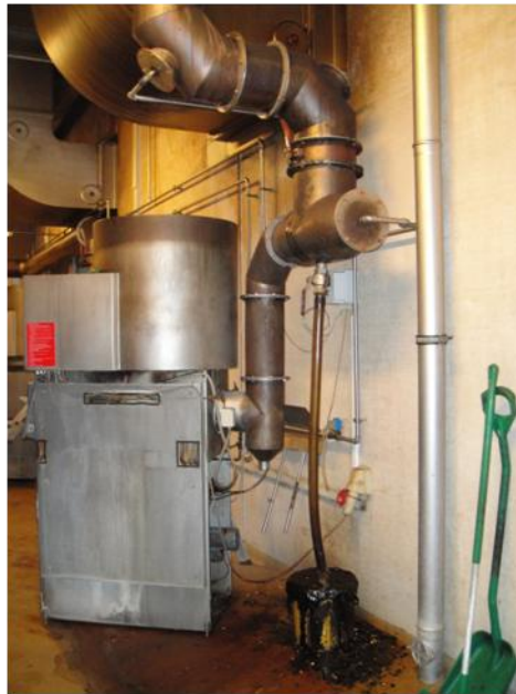
Smoke generator, notice the drain of soot from the exhaust.
