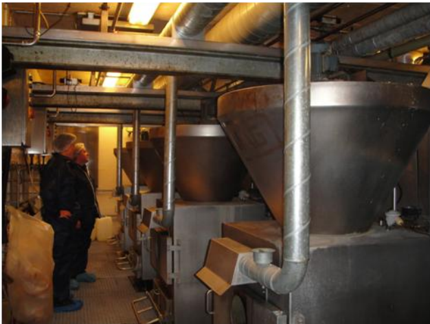
The line of smoke generators in one room.
