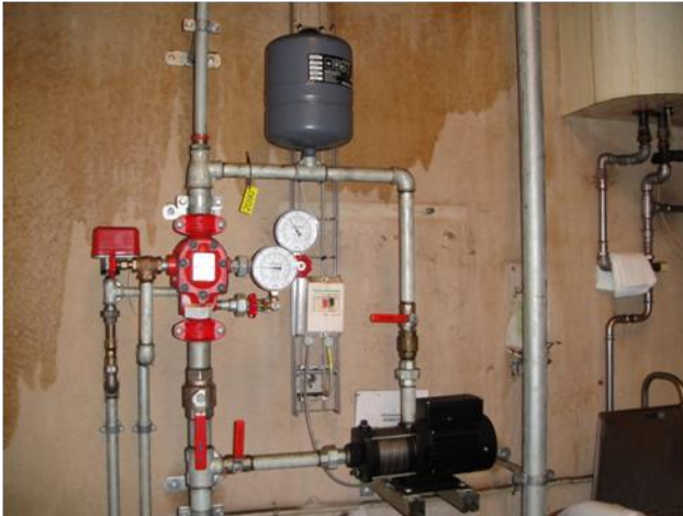
The systems pump station installed by DTEK
