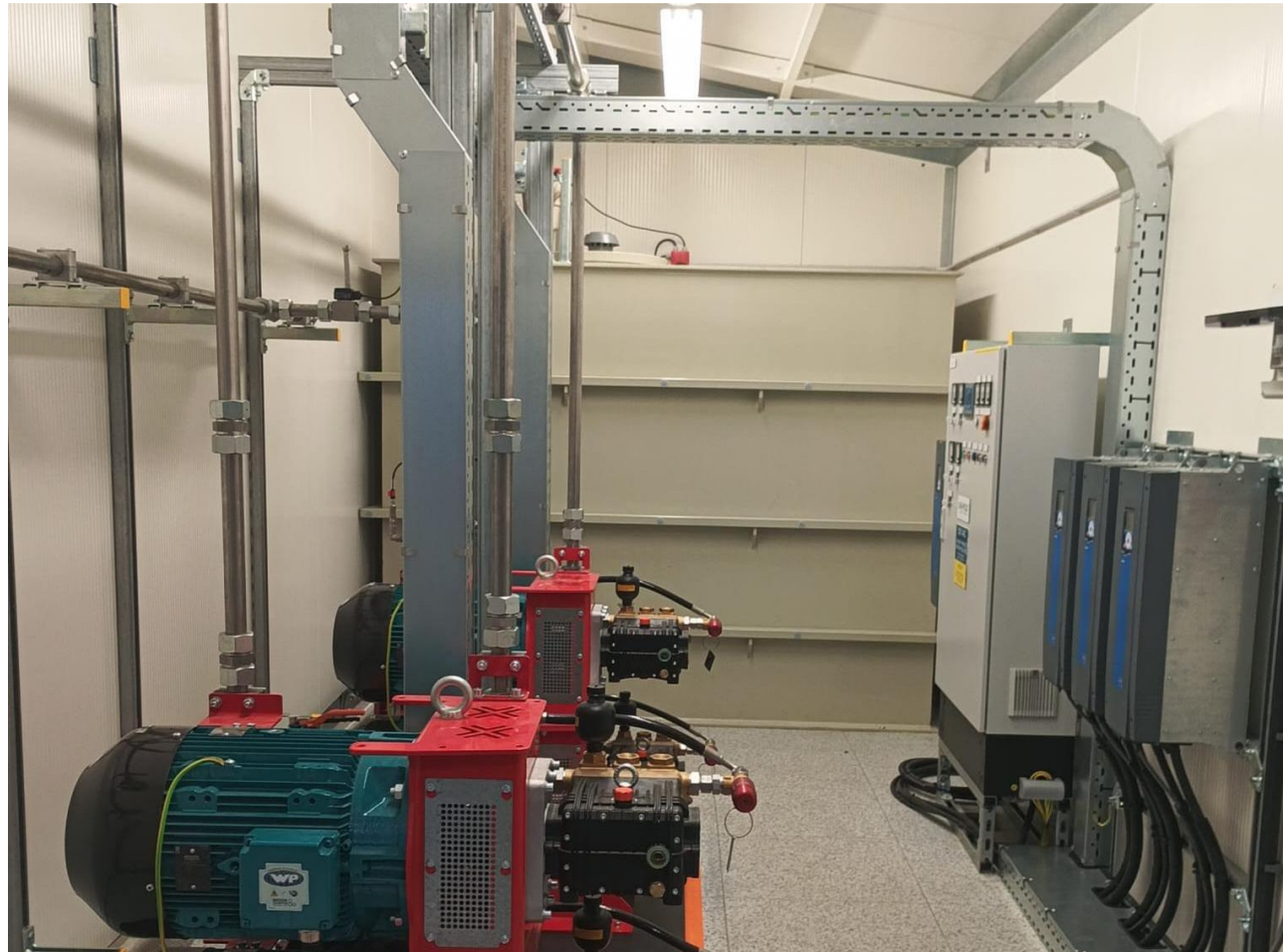
Project photo: LPU modules, stainless pipework and the switchboard/frequency converter side of the technological house.
