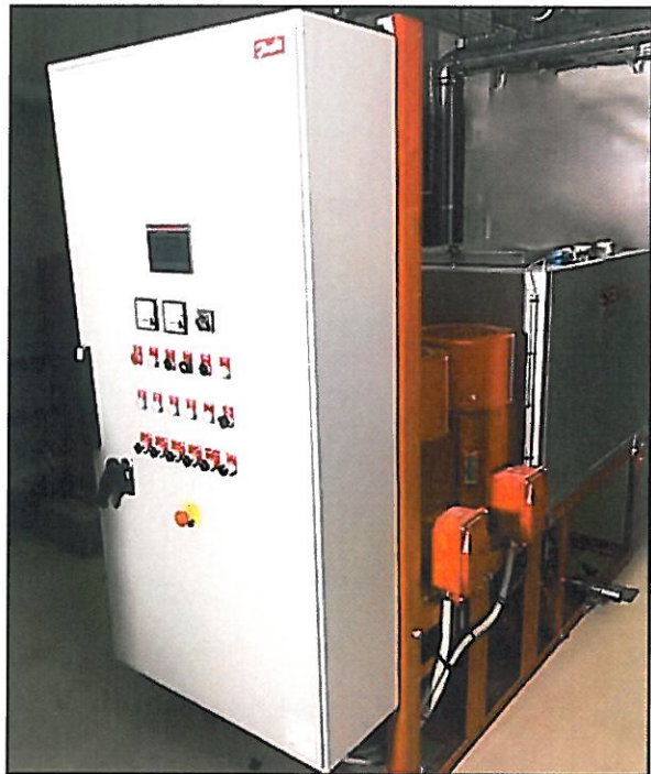
Control Panel Unit
